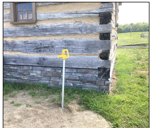
One of a dozen new hydrants added to our original four, not including the two at the public toilets. This one and one at Fort Tribute will be hidden by wooden well covers.
